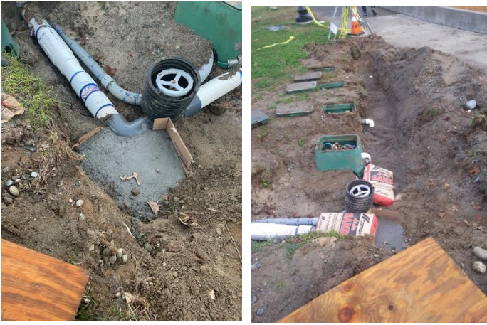
Repair to irrigation main service line at Riverbend Park (near North playground)
